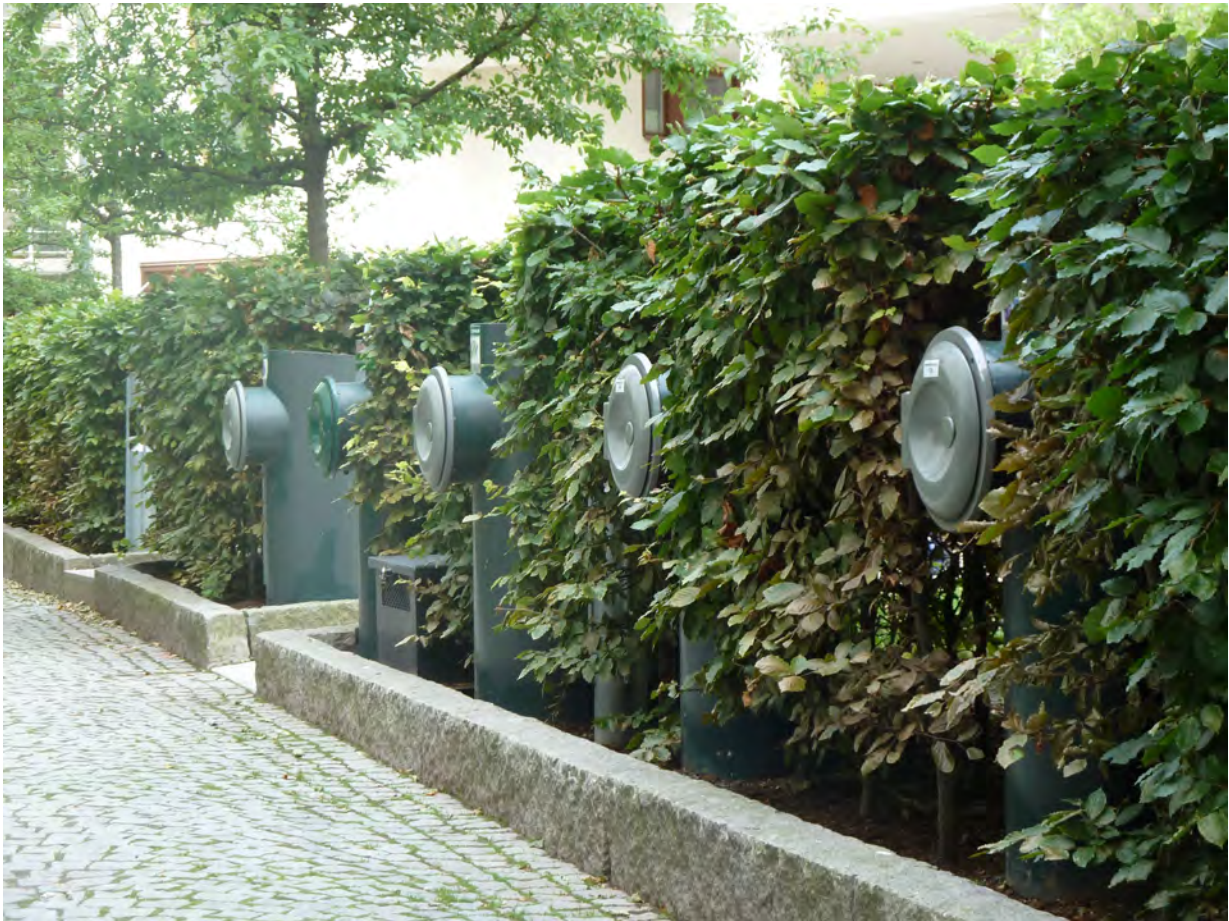
Integration of waste collection system into the green landscape of Hammarby Sjöstad. Photo: ©Françoise Labbé.
